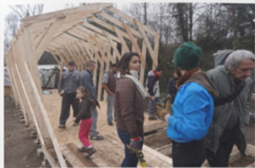
Constructing the PEROU Embassy in the shanty town of Rio-Orange. © Chloé Boleat
